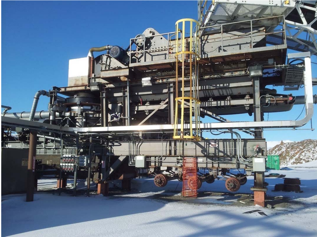
Figure 17-5 Secondary Crusher and Vibrating Screen
