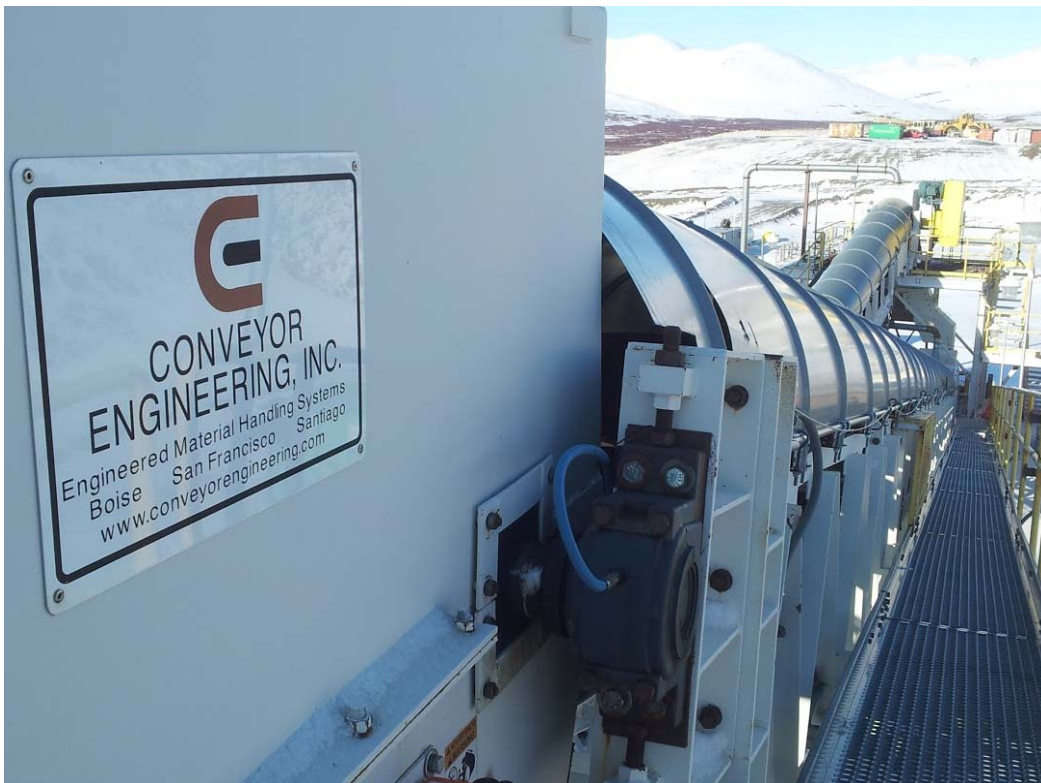
Figure 17-6 Recirculating conveyor in Tertiary Crushing Stage
